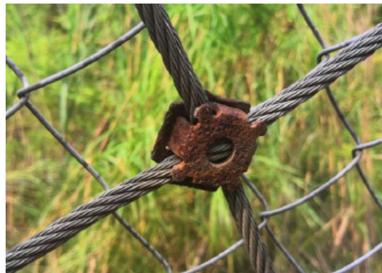
Figure 2. Cross buckle corrosion.
