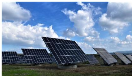
Figure 2 Miroslava PV power plant.
