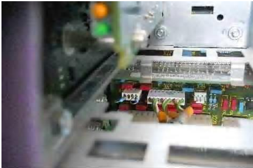
Figure 9. Inverter IMPI board.
